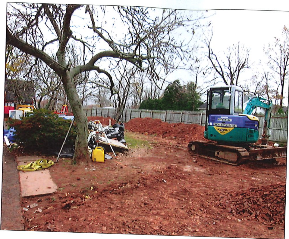
Many construction projects don't consider soil or tree preservation, which often necessitates soil remediation programs.
